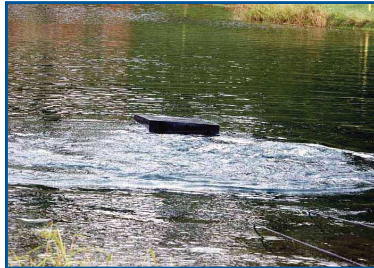
1/2 hp circulator moving water both horizontally and vertically.
