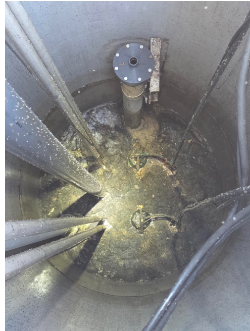
Mandeville Lift Station 27 before treatment
